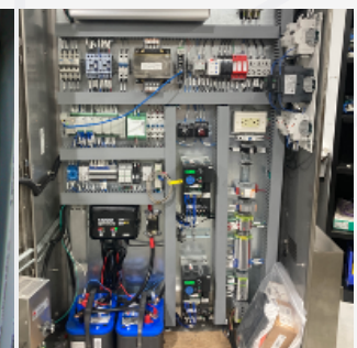
2024 Barrier Control Cabinet with BBU
